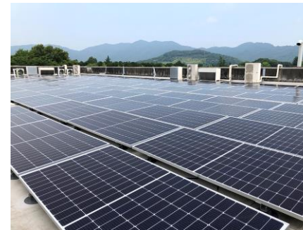
Solar power systems installed at Tochigi Plant
