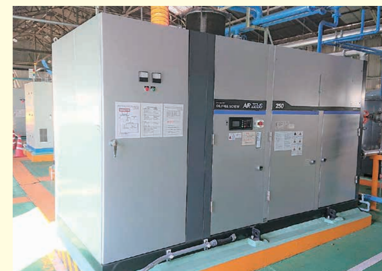
High Efficiency, Auto Controlled Air Compressor System Installed at Taga Factory
