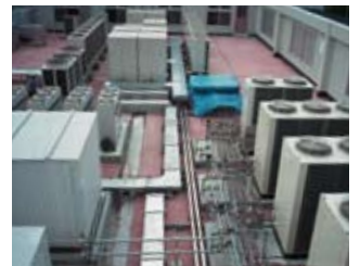
Ice thermal storage facility
