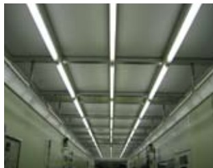
Laminar flow type clean room facility
