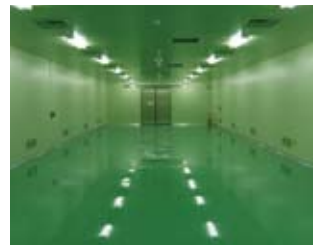
HACCP* clean room facility
