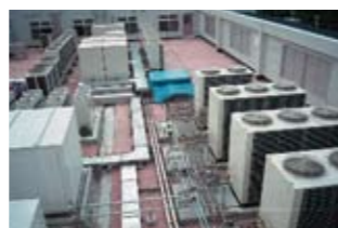
Ice thermal storage facility
