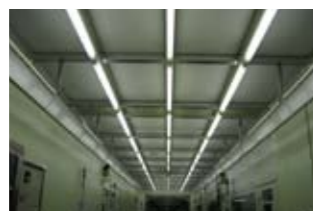
Laminar flow type clean room facility
