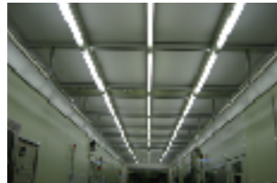
Laminar flow type clean room facility
